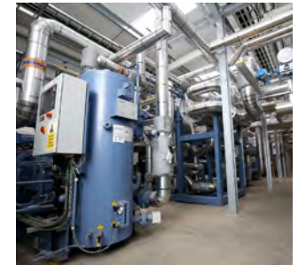
Mine Water Heat Source supplying GB Lubricants
